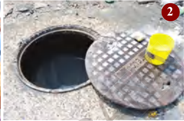
Manhole kept open on a road
